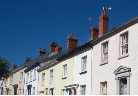
7 Stacks with matching details despite different size and most retaining matching pots
