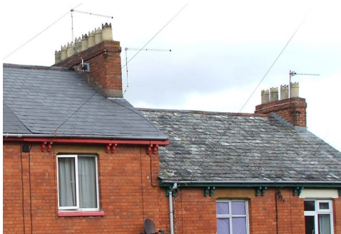
9 Banded stacks with chimney pots all matching style of pot generally found in Crediton
