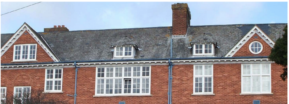
3 Early 20th century with variety of dormers including large gables and small hipped dormers
