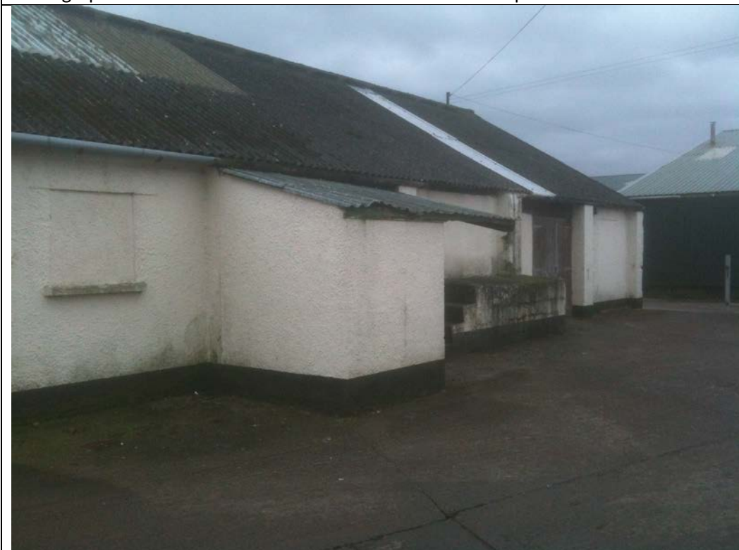
Photograph 2: An example of the older farm outbuildings with possible asbestos bound cement roofing.
